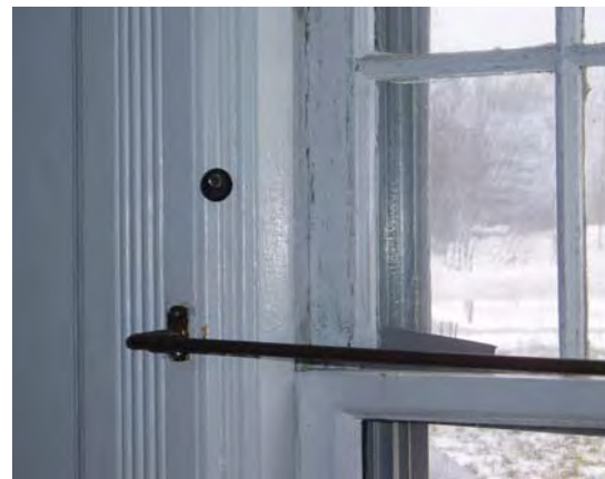
Window detail showing old glass in upper sash.
