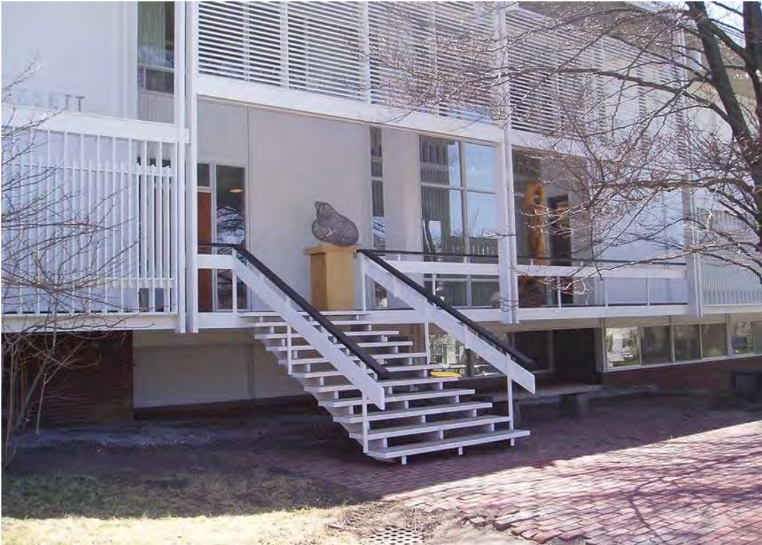
Detail of front (west) entrance with floating stairs, louver screens, and cantilevered porch deck.
